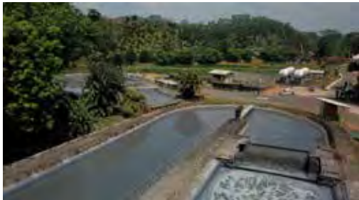
Effluent treatment plant
