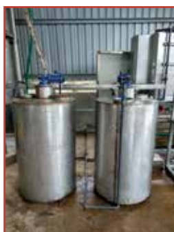
Chemical Mixing and Dosing Unit
