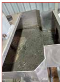
Sludge Mixing Tank
